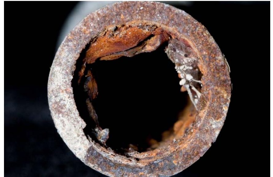
6 o'clock groove corrosion
